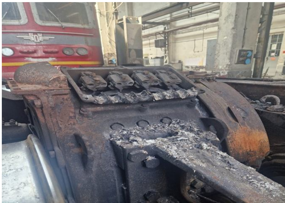
Fig. 4.9. View of second traction motor
