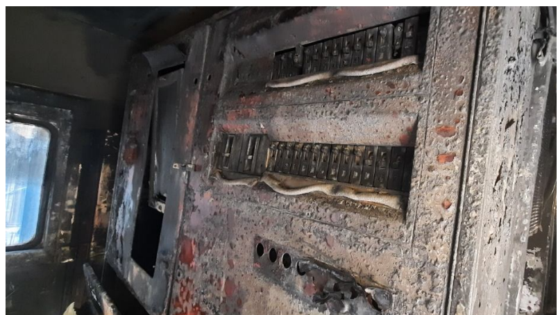
Fig. 4.12. Condition of the fuse panel in control cabin No. 1 after the fire
