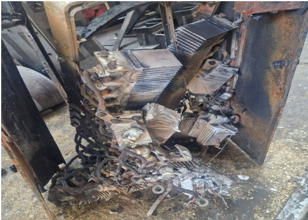
Fig. 4.5. View to the second rectifier block 022 and 221
