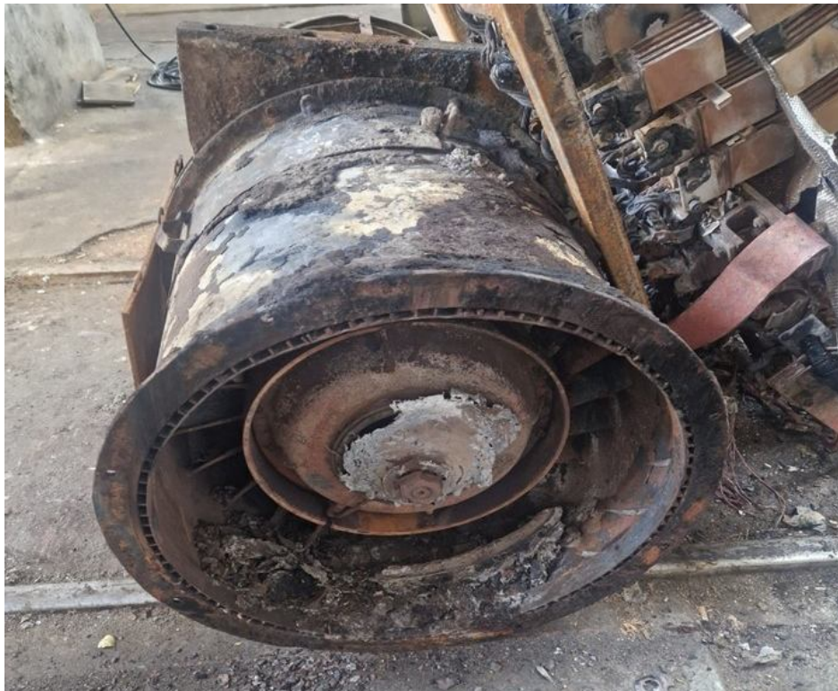
Fig. 4.10. View of the horizontal fan after the fire
