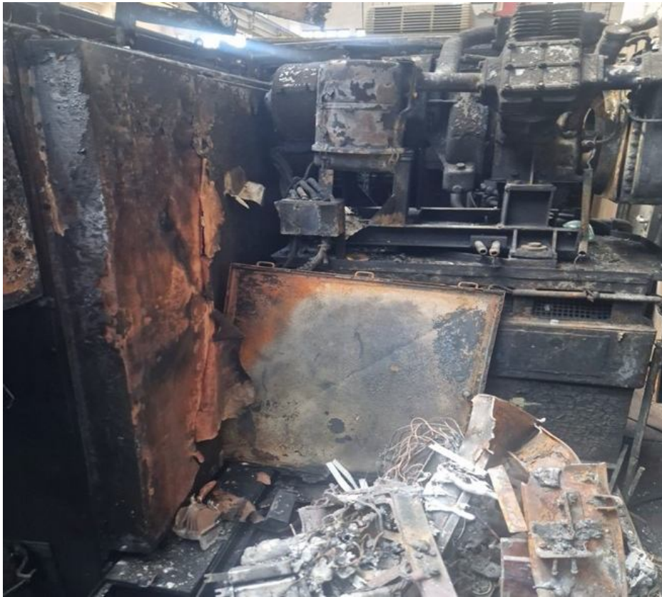
Fig. 4.6. View of the burned rectifier 022 and 221
