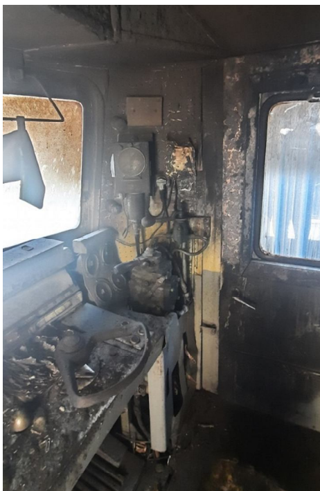
Fig. 4.11. Condition of the control cabin № 1 after the fire
