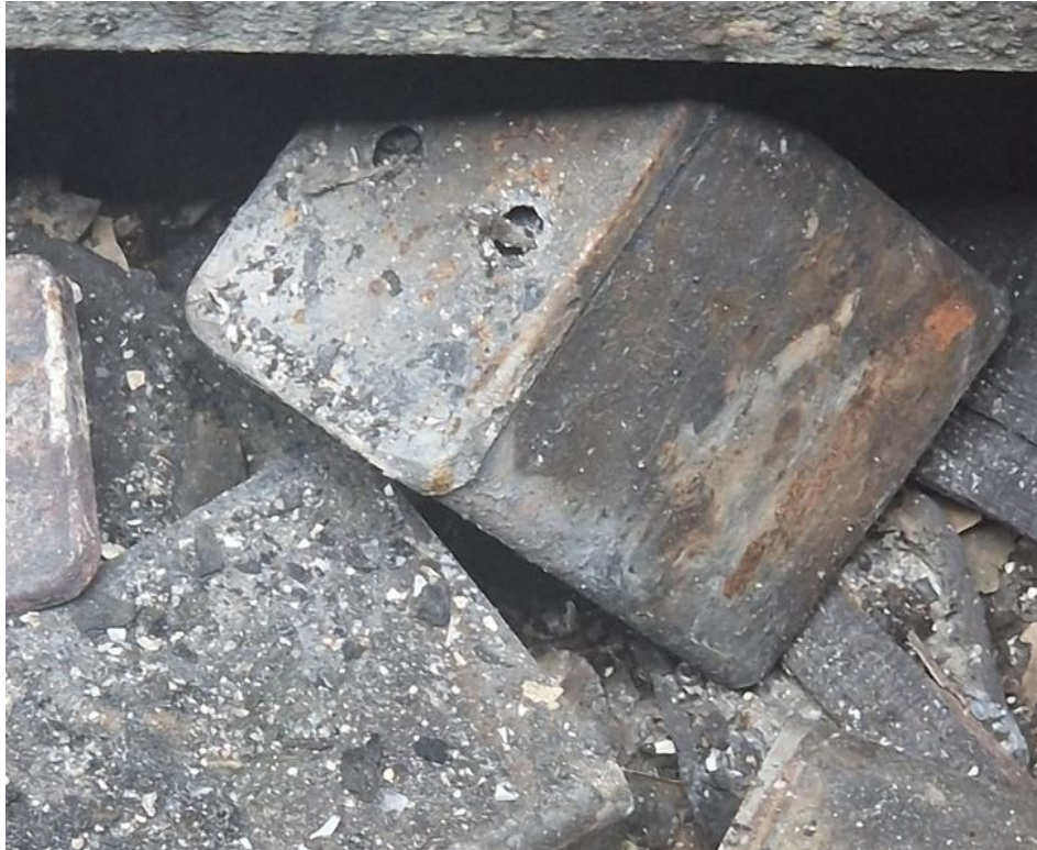
Fig. 4.8. View of blasted capacitor of R-C groups of 221
