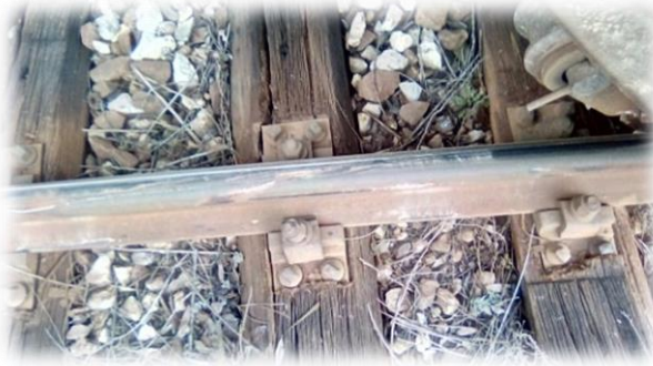
Figure 4.2.8.5: Appearance of the pockets of rotten sleepers
