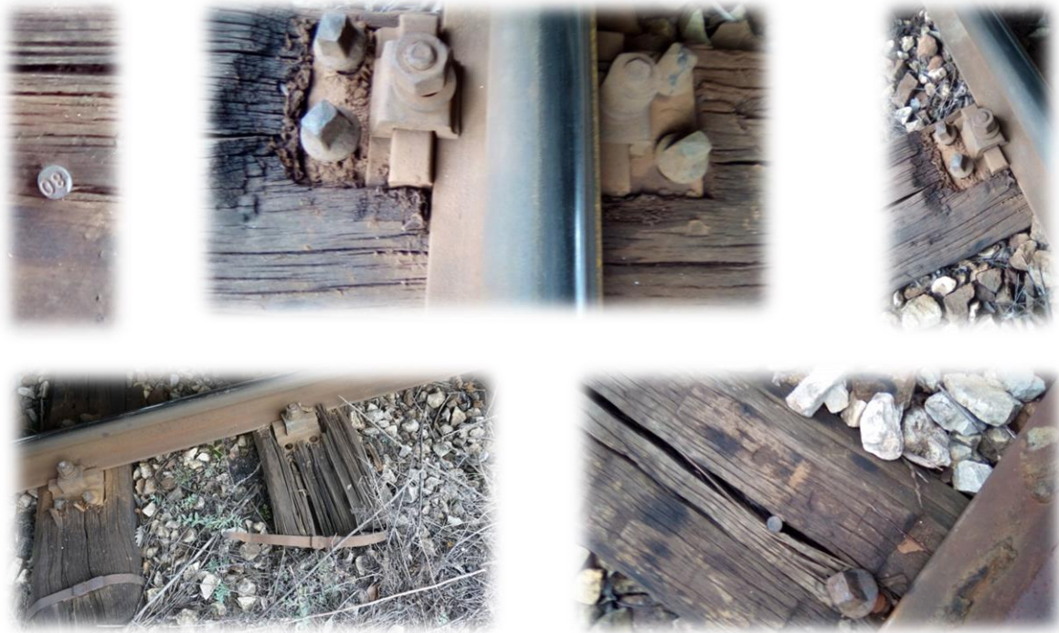
Figure 4.2.10.3: Local decay beneath the rail support and longitudinal cracks in the sleeper.
