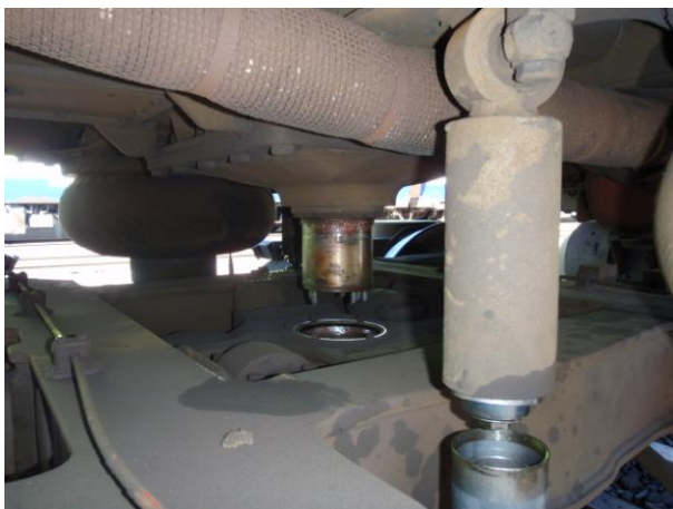
Figure 7 – Failed bogie to carbody connection
