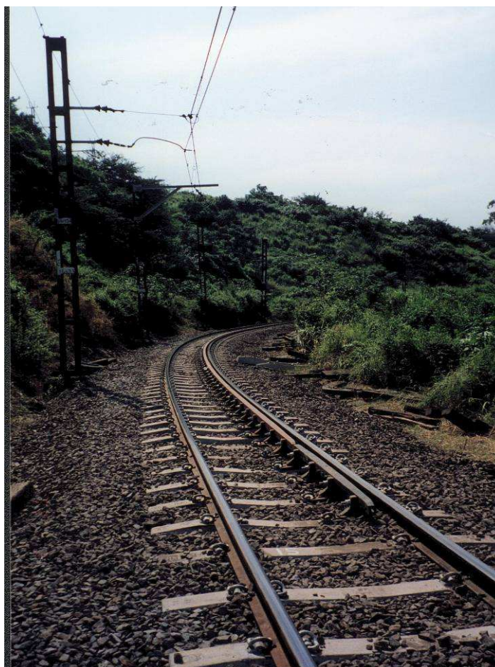
Figure 7: Example from RSA showing Check Rail installation in Curved Track
