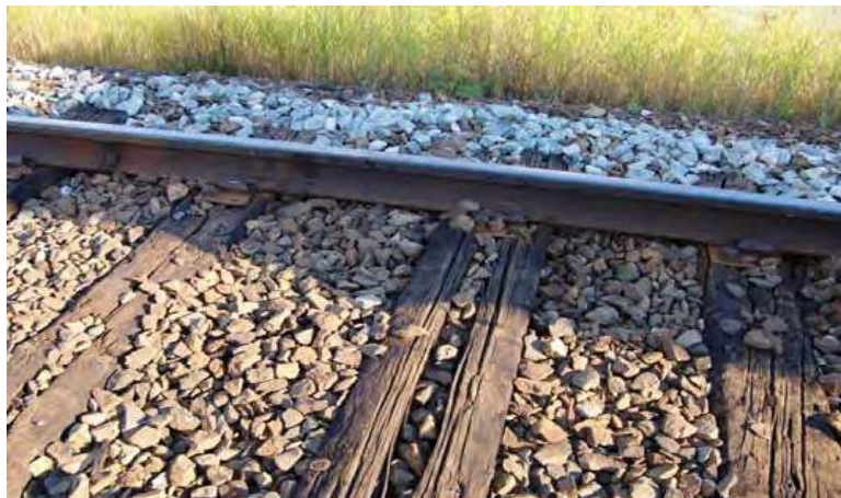
Figure 4: Example of a Track Width Failure 7
