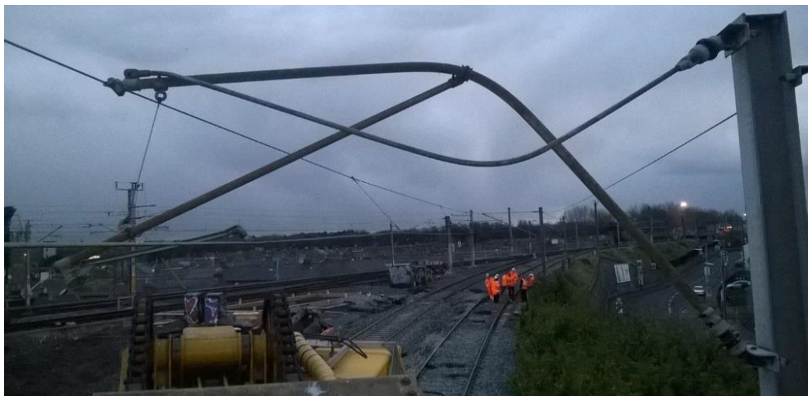
Figure 26 – Damage to the cantilever
