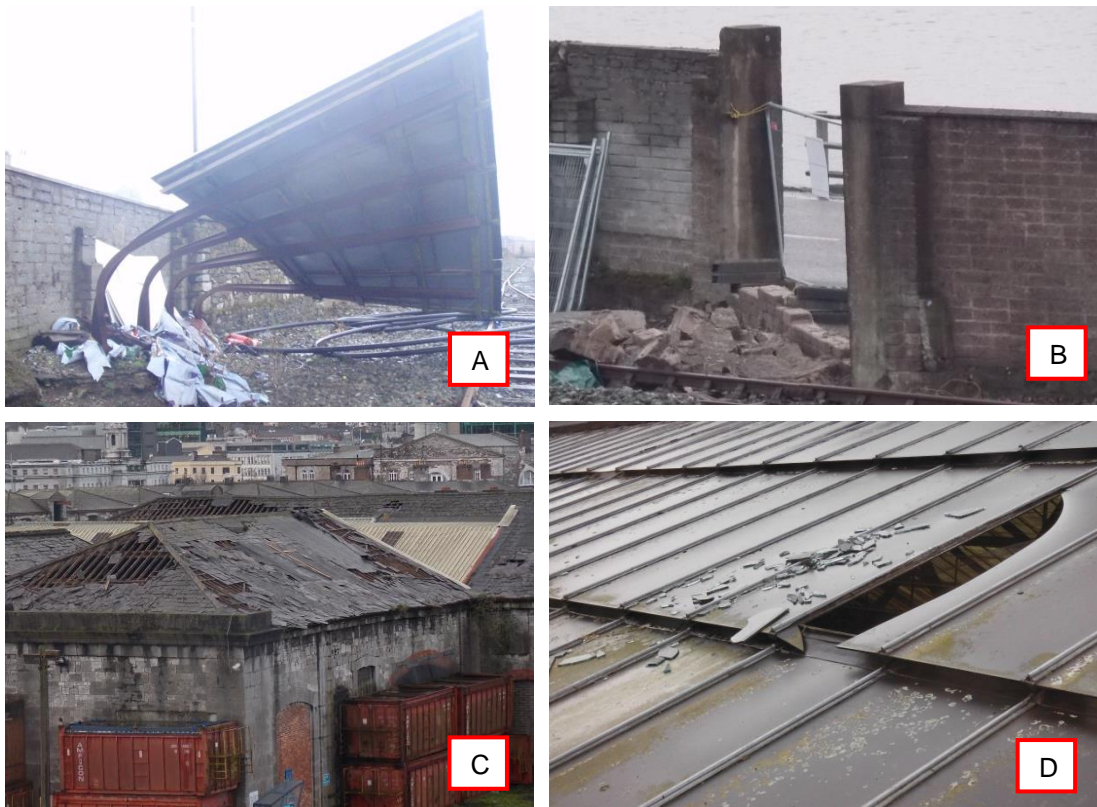
Figure 7 – Additional damage in vicinity of Kent Station
