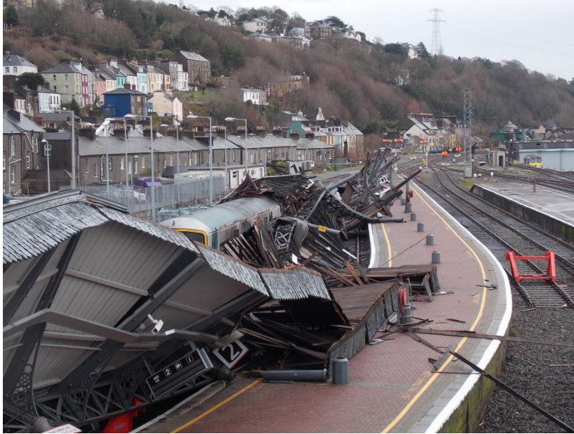
Figure 2 - Collapsed canopy and resultant debris
