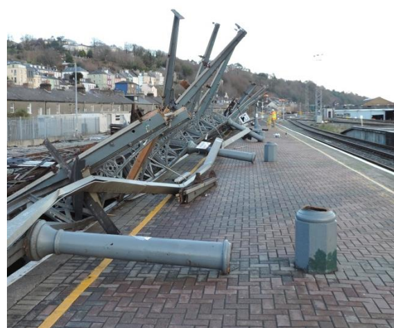
Figure 17 – View of collapsed canopy
