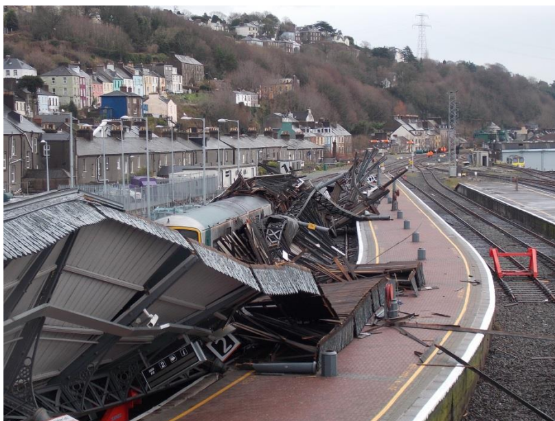
Figure 6 – Collapsed canopy and resultant debris
