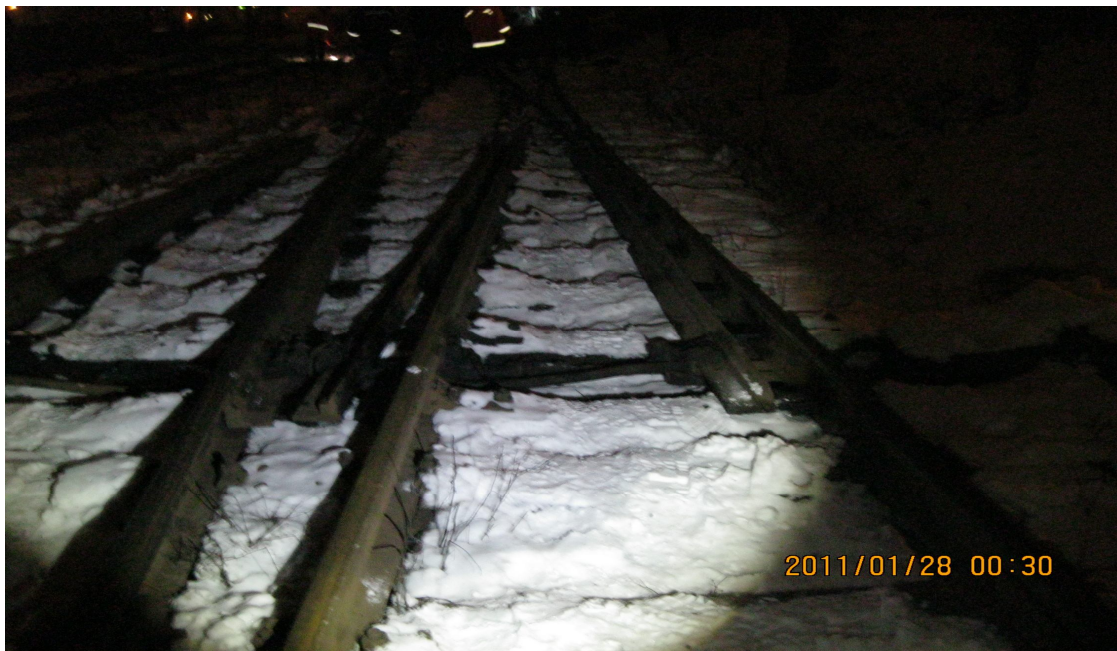
Fig.2 Switch no. 7 in TDJ 3/7
