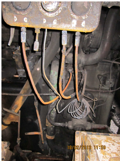
Photo no. 2 The devices area from the damaged engine room
