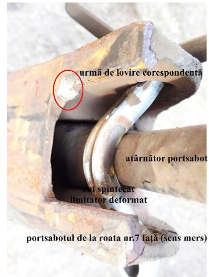
Foto nr.3 – hit mark on the brake shoe holder of the corresponding wheel nr. 7
