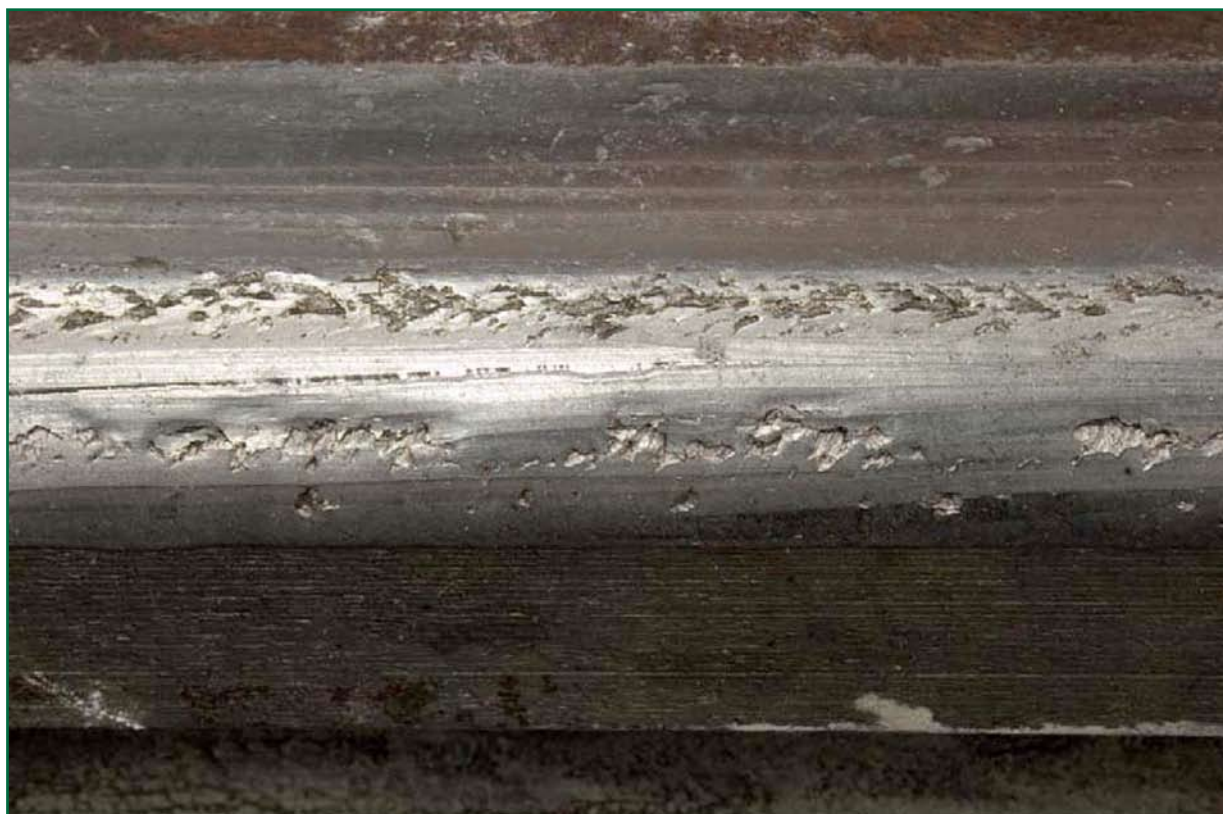
Figure 10: Rolling contact fatigue marks on the switch rail, overlaid by wear on the gauge corner.
