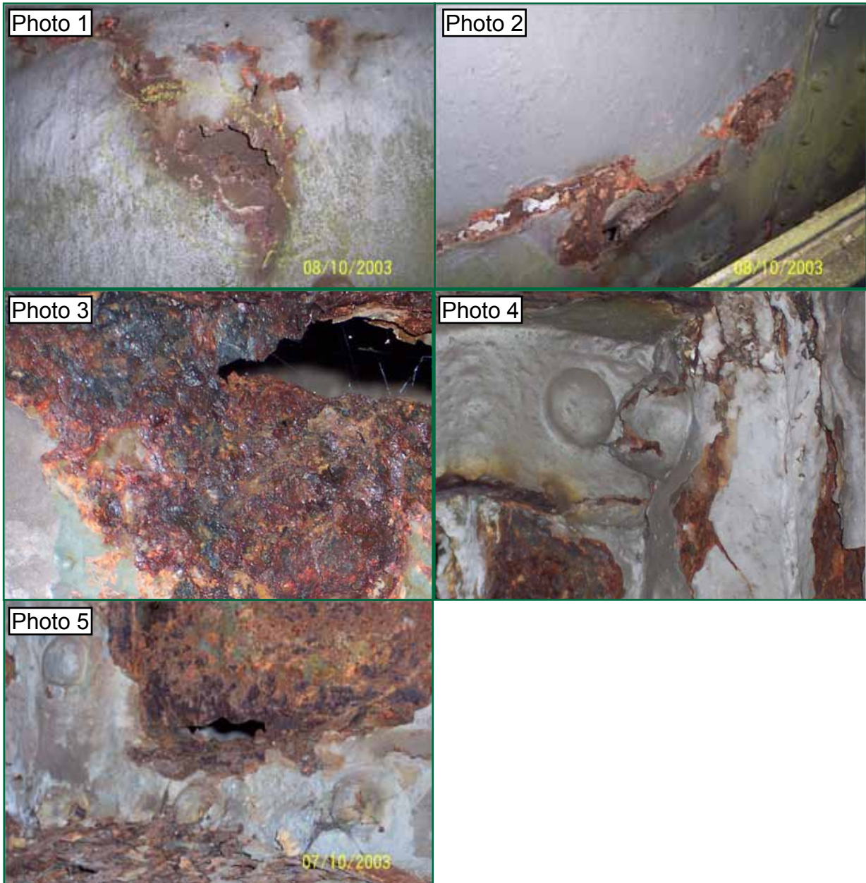
Figure G1: Photographs from Atkins urgent defect report (photographs courtesy of Network Rail)
