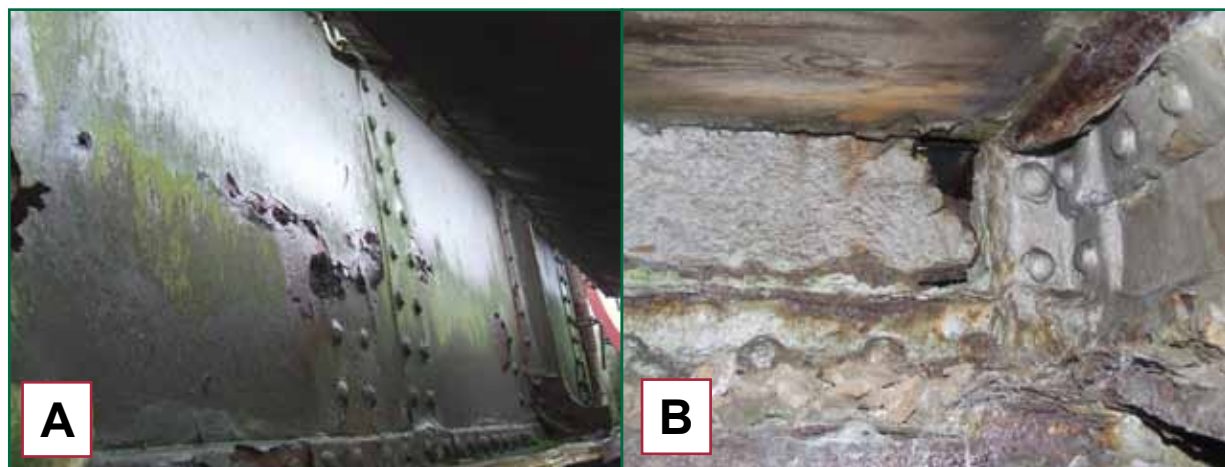
Figure 23: Photographs of web corrosion from the Inspection for Assessment undertaken 27 November 2007 (photographs courtesy of Network Rail)
