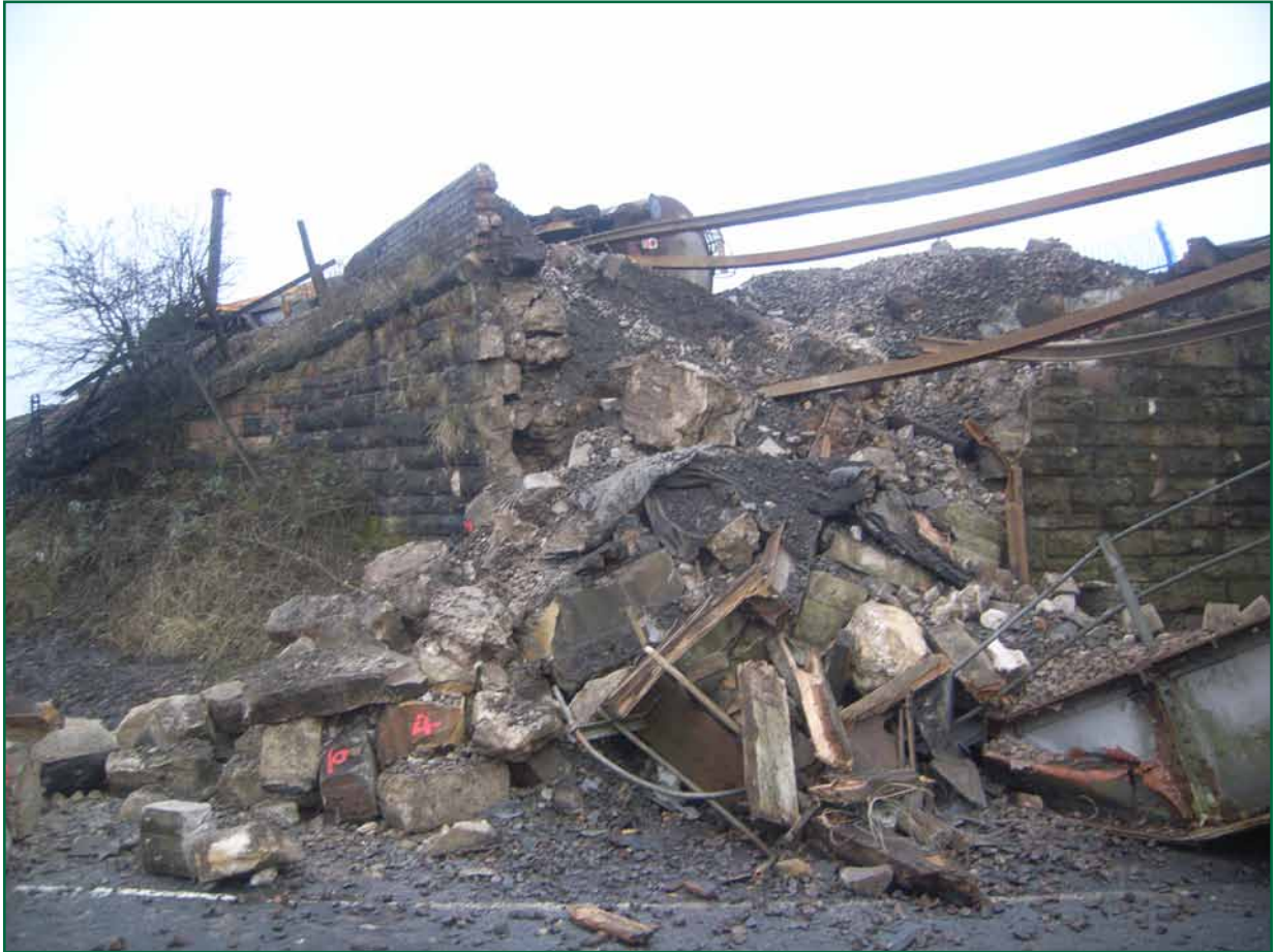
Figure F4: Photograph of debris from failed south abutment
