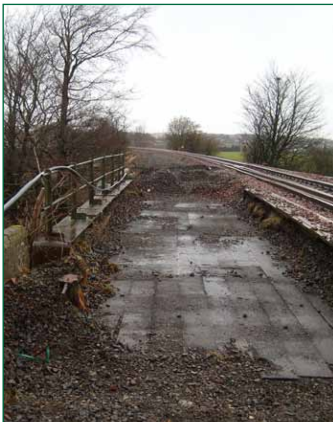
Figure F3: Site photograph of the west deck after the ballast was removed on 16-17 January 2009 (photograph courtesy of Network Rail)
