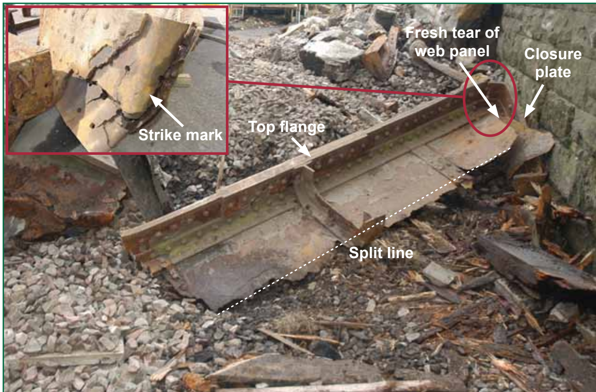
Figure 12: Upper part of the south end of the centre main girder showing the horizontal split line, the folded closure plate and fractured flanges (main photograph courtesy of British Transport Police)
