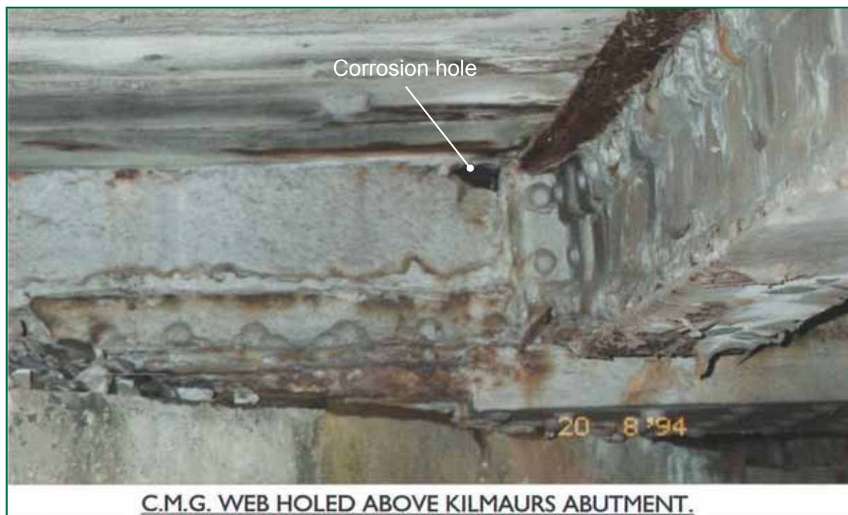
Figure 21: The web plate corrosion hole at the south end of the centre main girder that was illustrated in the 1994 Assessment report (photograph courtesy of Network Rail)
