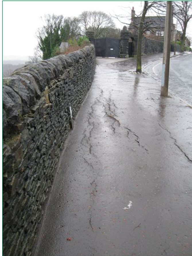
Figure 9: Pavement cracks behind a different section of the wall after the derailment (courtesy of Network Rail)
