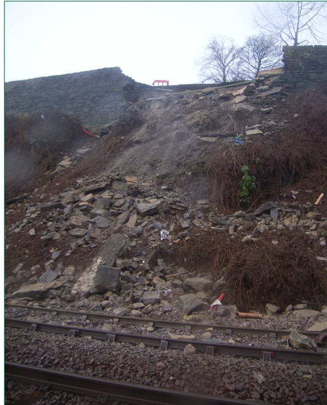
Figure 4: Collapsed section of the wall
