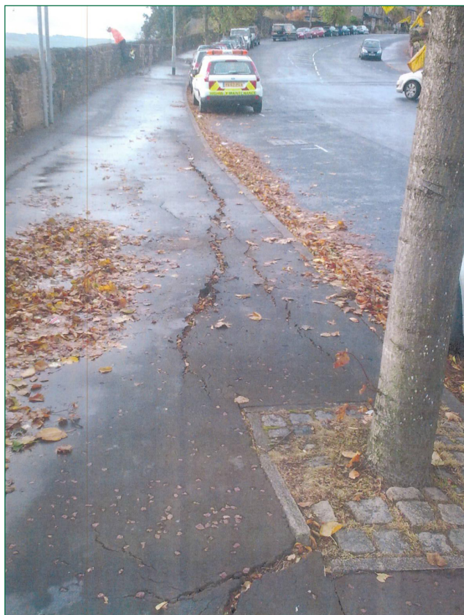
Figure 6: Pavement behind the wall in October 2010 showing cracks (courtesy of Calderdale MBC)
