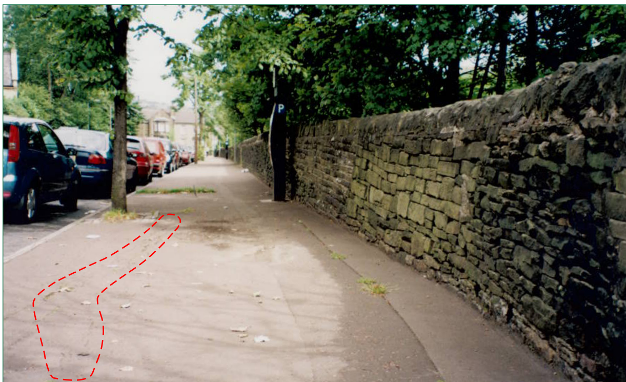
Figure 5: Pavement behind the wall in 2003 showing cracks (highlighted) from 2003 detailed exam report (courtesy of Network Rail)
