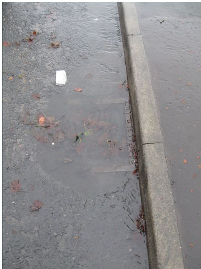
Figure 8: Road drain in Dudwell Lane shortly after the derailment (Courtesy of BTP)
