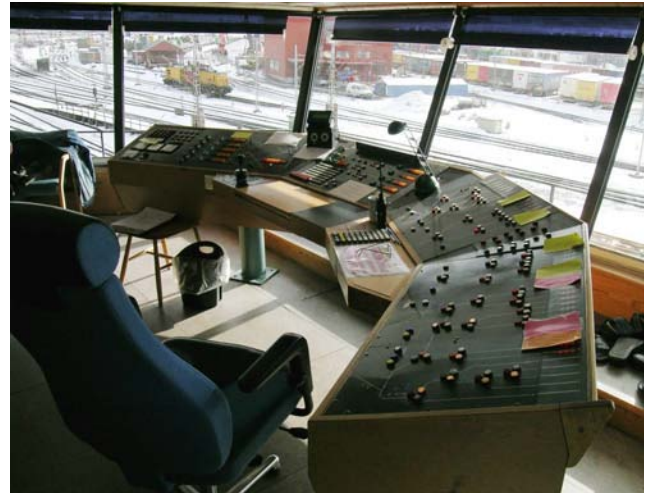
The workplace in the slip signal control centre. The control panel for the brakes on the left.
