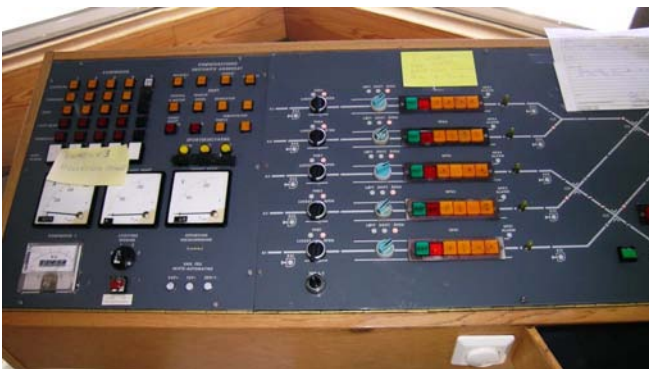
Figure 3: The control panel for the brakes.
