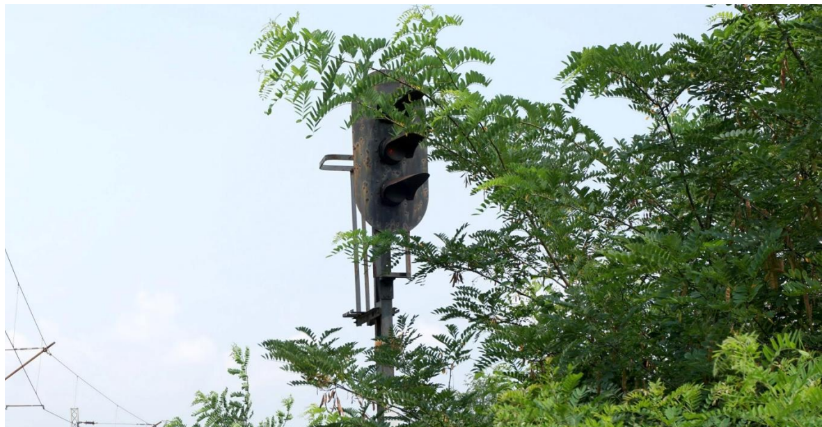
Fig. 4.1.5: Appearance of the automatic block signal E 51
