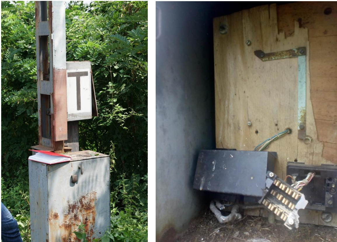
Figure 3.4.3.1: External and internal appearance of TT cabinet on the pillar of the automatic block signal E 51
