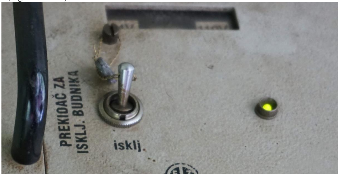
Figure 3.4.4.1: View of the switch of the electronic part of the driver's safety device on the locomotive. 661-162
