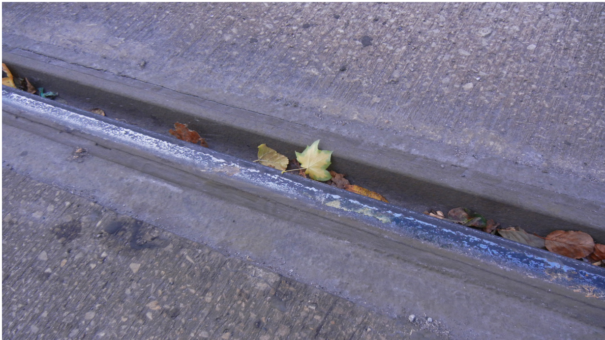
Figure 11: Photograph of rail head at Shalesmoor, taken immediately after accident. Note that rail head is black in colour and the presence of fallen leaves
