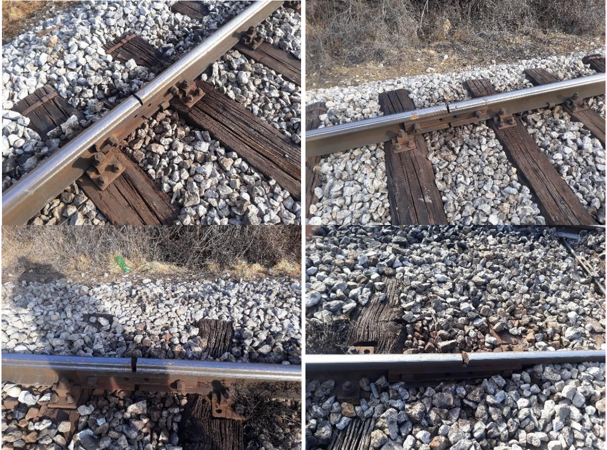
Figure 4.2.9.7: The appearance of railway joints in the broader area of the serious accident (floating unbalanced joints)
