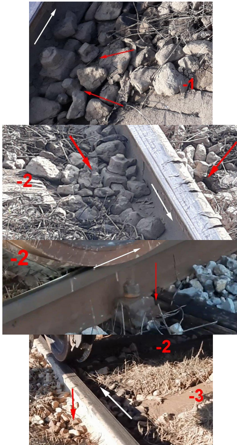
Figure 4.2.1.20: Condition of the fastening equipment in the zone of the first wheel derailment
