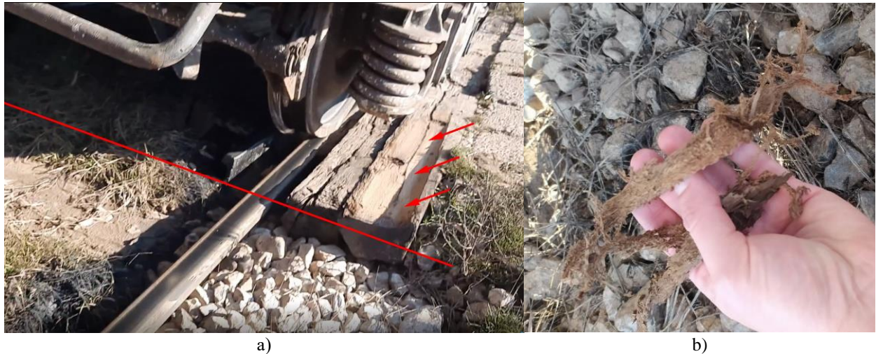
Figure 4.2.5.1.1: Hollowed part of the wooden roadway structure at the level crossing
