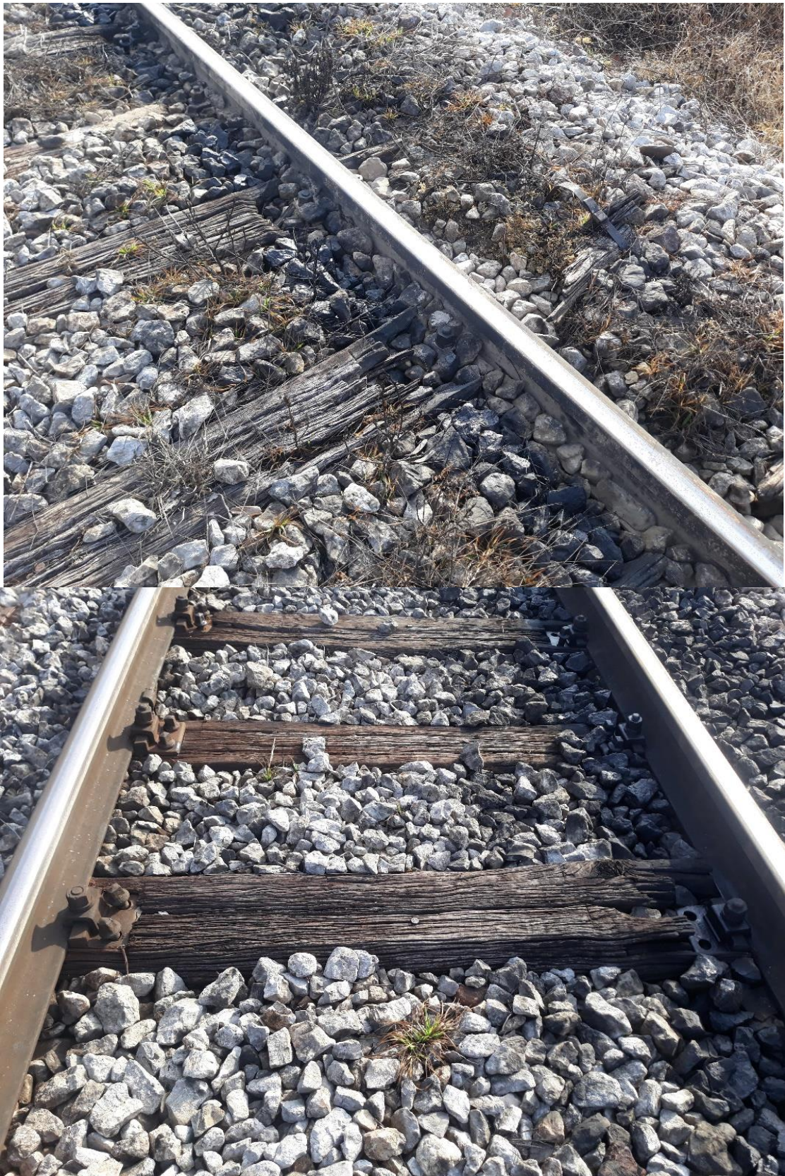
Figure 4.2.6.1: Appearance of the wooden sleepers in the serious accident zone (source: "IŽS" a.d.)
