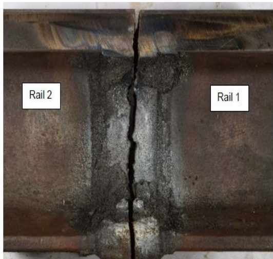
Figure 9 – Transverse failure through the centreline of the weld
