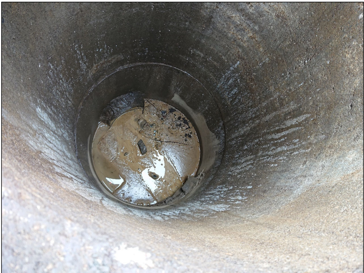
Figure 2: Blocked deep drainage pipe
