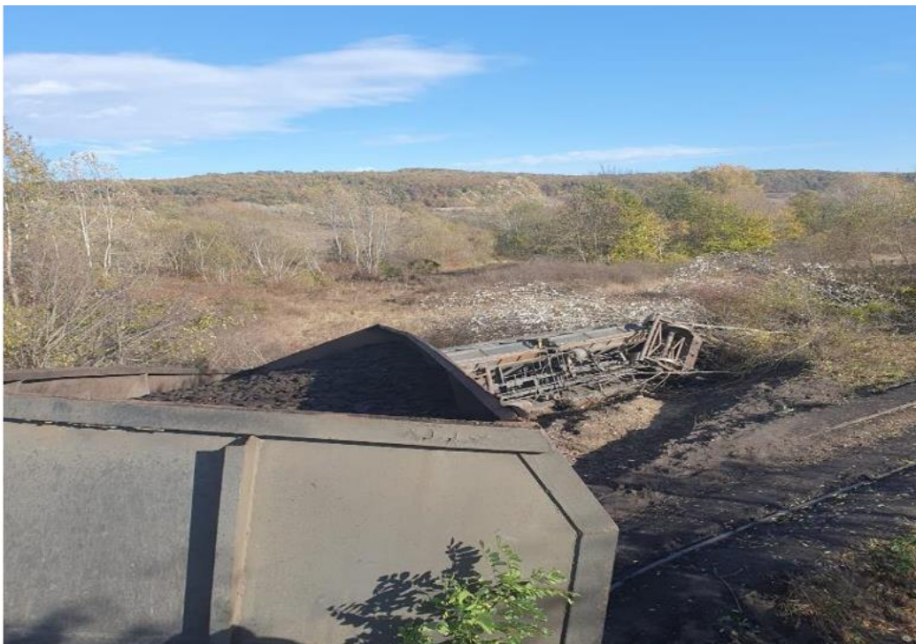
Photo no.1: First wagon overturned 12 m off the track and 2nd wagon derailed
